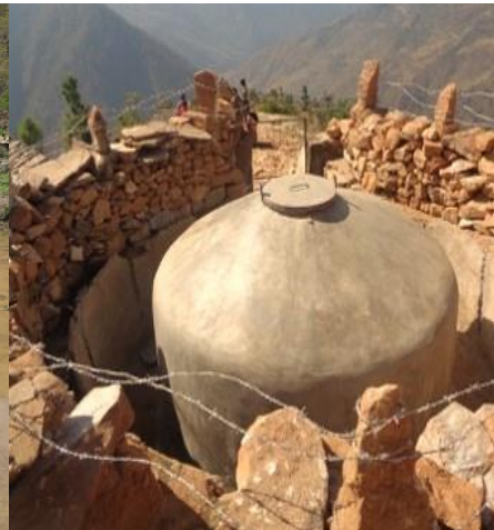
Rain water harvesting tank at Suwanauli VDC, Jajarkot
